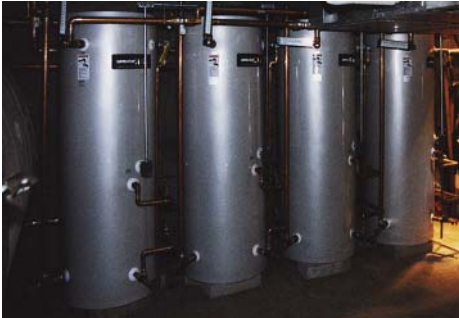
The more cost-efficient four 120-gallon tanks that replaced the failed 1,000-gallon tank.
