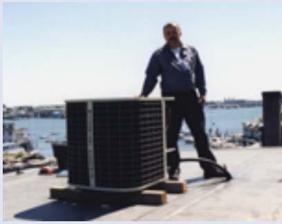
Air conditioning with a view.
